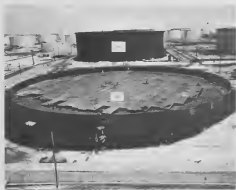
Four tanks in a row and two other new tanks in eastern Tank Farm are being built by Chicago Bridge. Tanks 764 and 765 are in background. Eight other tanks are also under construction for the HDS project.
